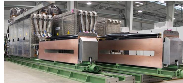
Slab Induction Heating Coils
